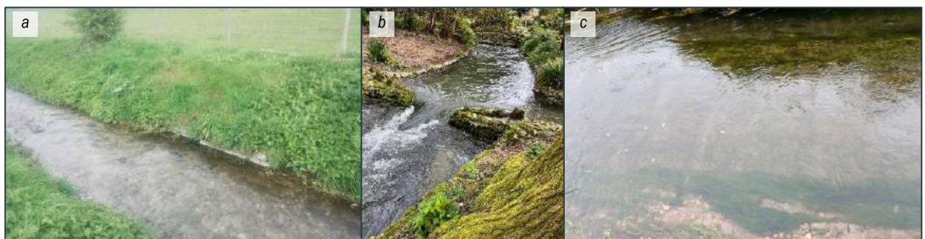
Plate 10 a) small bank toe reinforcements (RL03), b) major bank and partial bed reinforcements (RL10a); c) bed reinforcements associated with old footbridge (RL18)
