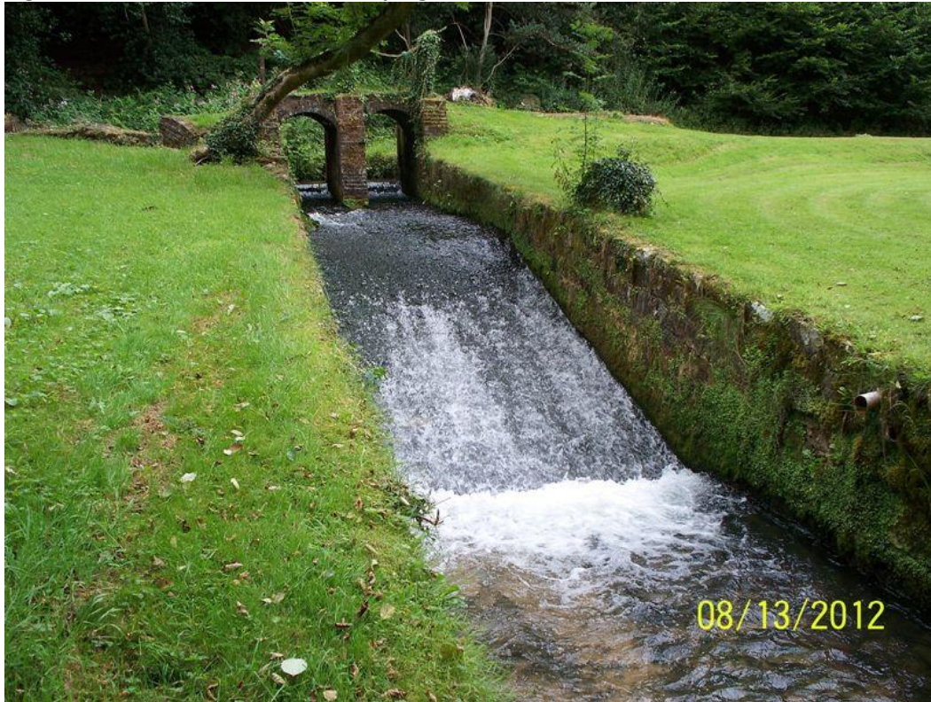
Figure 2: Before the works - the sloping weir built within the stone mill leat on the Costers Brook
